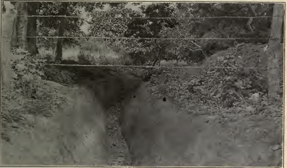
GOOD EXAMPLE OF "V" TYPE DITCH WITH SLOPE SLIGHTLY STEEPER THAN 45 DEGREES
